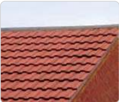
No chimney or flue
